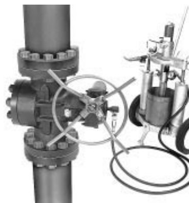
Pneumatic sealant gun (5 quart size) being used to lubricate 6" early design Super-H valve with the sealant fitting on top of the stem.
