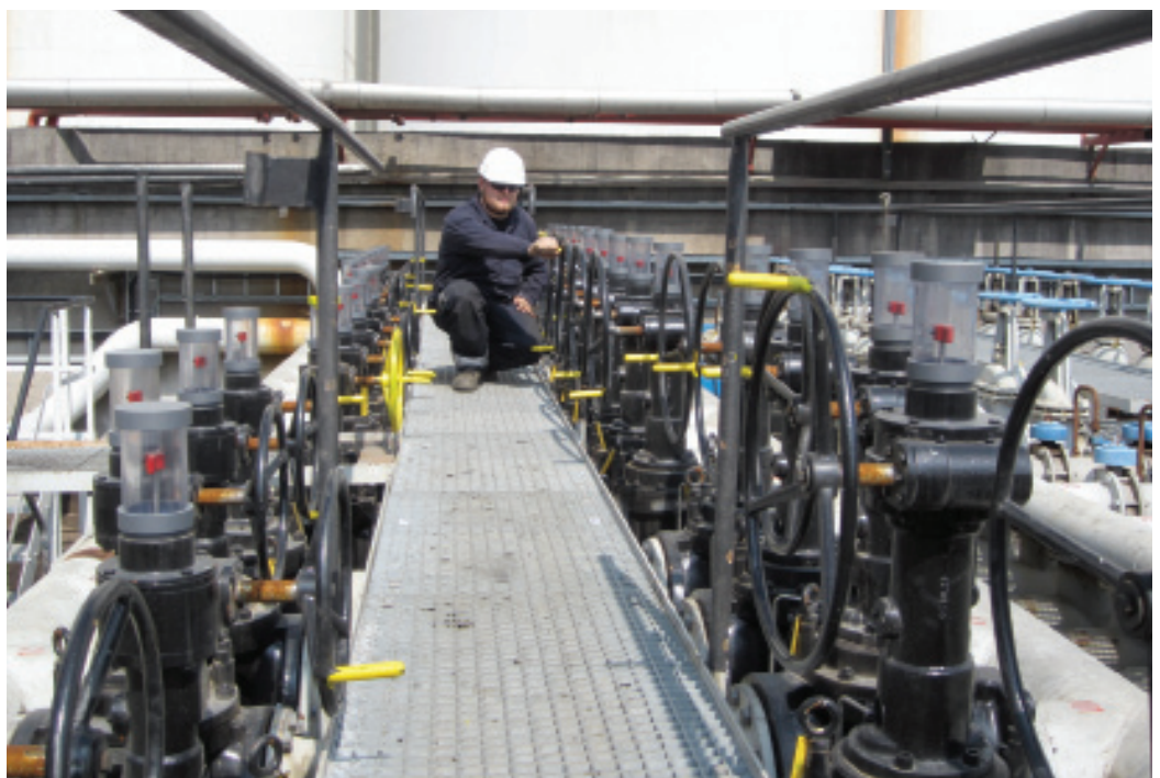
Engineering supervisor Søren Lorentzen operating one of the Omniseal DB&B expanding plug valves at OTC
